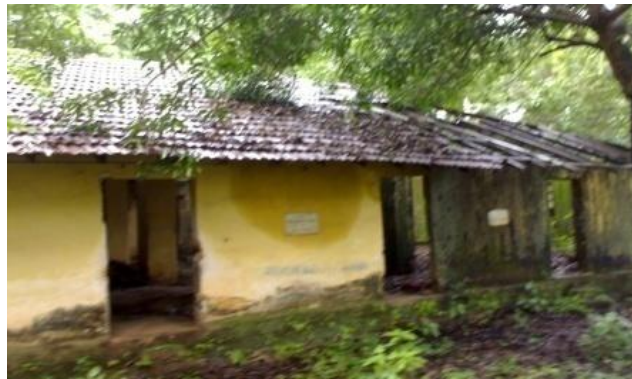
Dilapidated condition of leprosy hospital
