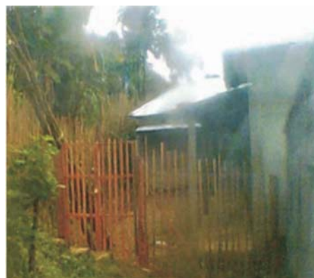
Boundary wall at Lawngtlai-I Primary School constructed by private unregistered contractor during 2010-11
