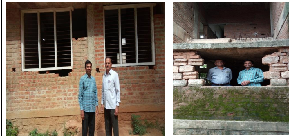
Exhibit 1: Incomplete BEO Office building at Tumakuru (31.8.2017)
