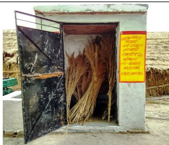
Plate 5.2: Non-functional toilet GP-Kirachan, Block Rajepur, Farrukhabad, Uttar Pradesh
