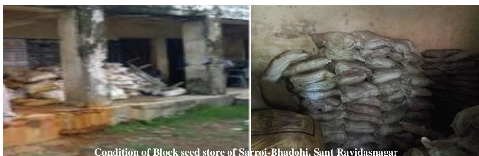
Condition of Block seed store of Sarroi-Bhadohi, Sant Ravidasnagar
