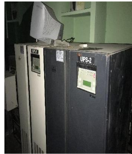
Online UPS remaining non-functional at Northern Region, Malda
