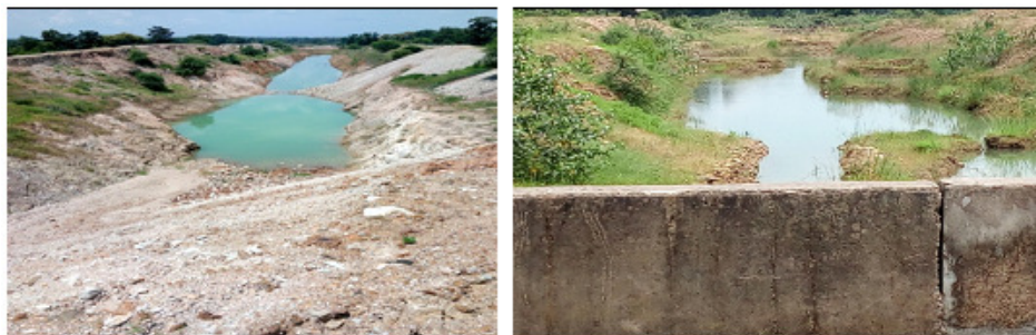
Photographs showing damage to work executed on the project
