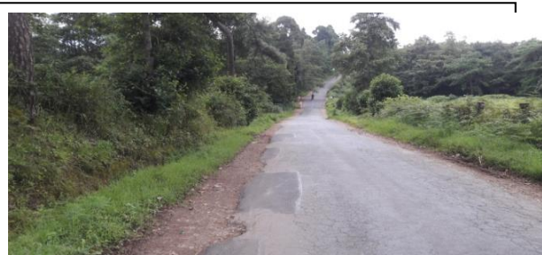
Picture showing the repair work undertaken (Nov – Dec 2017) at a cost of ₹1.70 lakh after the work 'Widening i/c MBT of existing pavement of Shillong Peak Road - under RIDF-XX' which was completed in December 2016. Date of joint physical verification: 07.08.2018
