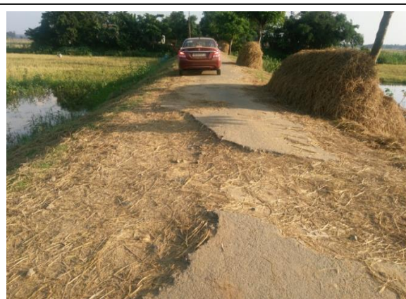
Picture showing broken road in the work 'Improvement i/c MBT of a road from AMPT road to Haribanga village via Bholarbita (0.300 Km) under RIDF-XX' which was completed during February 2017. Date of joint physical verification: 05.06.2018
