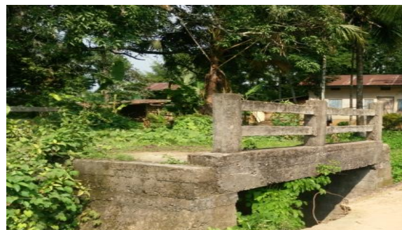
The work 'box cell culvert' against the main work 'Improvement i/c MBT of a road from Gimigre Old Model to Bollochiring (0.00-2.00km) under RIDF-XX' constructed at a cost of ₹ 13.76 lakh remained unutilised as the approach road could not be constructed due to land dispute. Date of JPV: 05/06/2018
