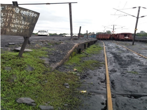
Pic. 03: Para No. 4.6.1, Table No. 06, Sl. No. 04: Jarangdih Railway siding of CCL without fixed sprinklers
