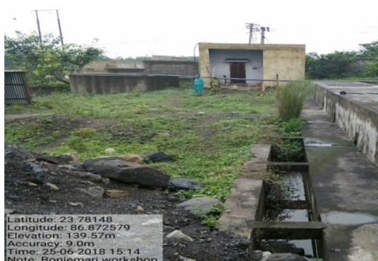
Pic. 06: Para No. 5.5.1 (Sl. No. 01): Existence of weeds in HEMM washing facility at Dabor, ECL
