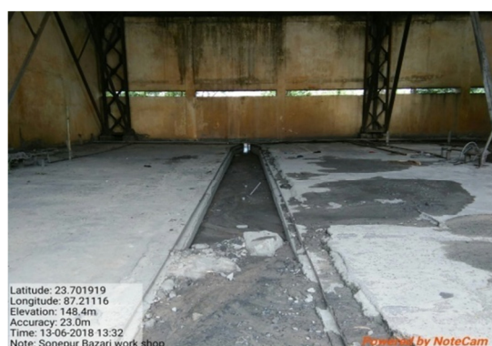
Pic. 07: Para No. 5.5.1 (Sl. No. 02): Choked drains and chambers of HEMM washing facility at Sonapur Bazari, ECL, resulting in overflow of sludge
