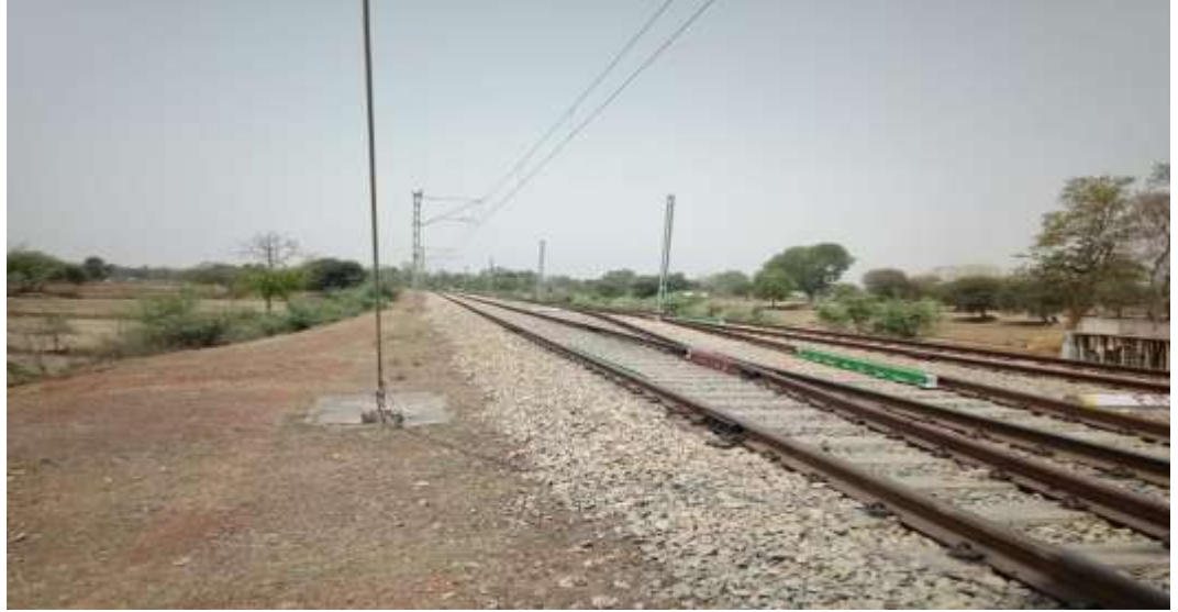
Incomplete wire stringing work
